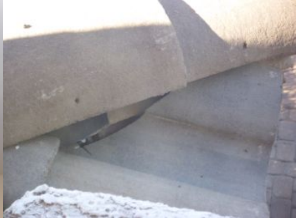
Improperly installed roof tile at hip in front
