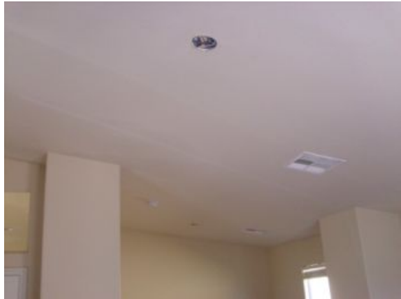
Exposed electrical wiring needs cover Master bedroom
