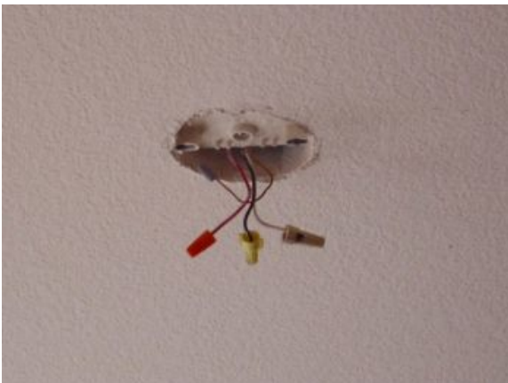
Bedroom 3 exposed wires on ceiling
