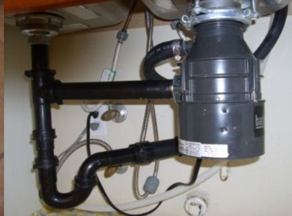
Jammed garbage disposal
