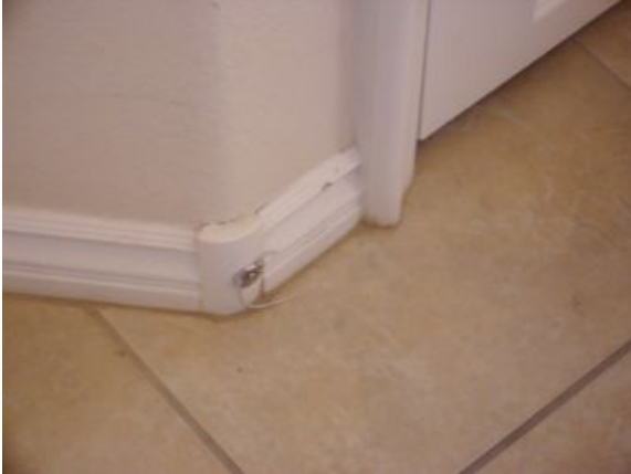
Broken door stop at door at bottom of stairs
