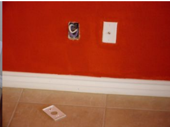
Missing cable cover
