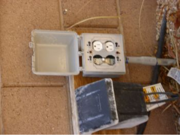
Switch incorrectly installed
