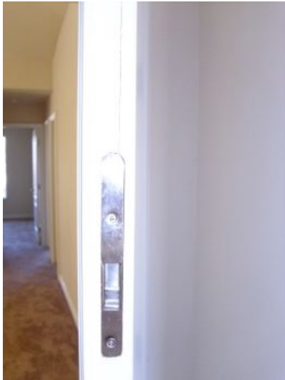
Master bedroom entry door has split in end of door
