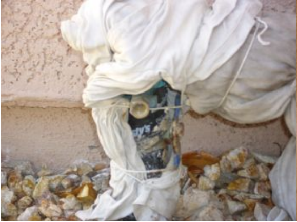
Gate valve corroded from leak
