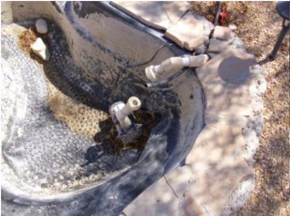
Disconnected water feature pump
