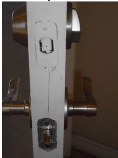
Fire door to garage has split in end of door
