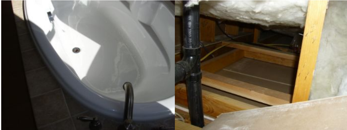
Master bath tub stopper missing
