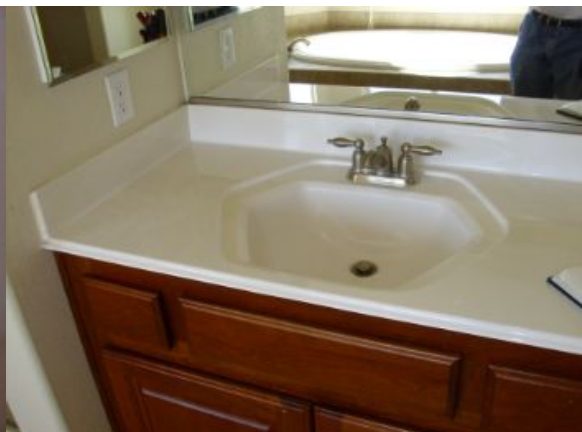
Master bedroom sink stopper not connected
